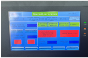
Touch Screen PLC
